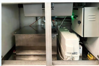
Water leak detection system 漏水偵測系統
